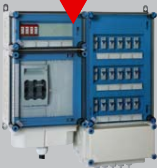
PV Solar inverter collector
