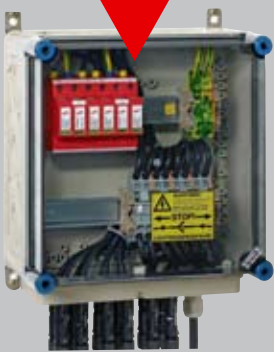
PV generator junction boxes
